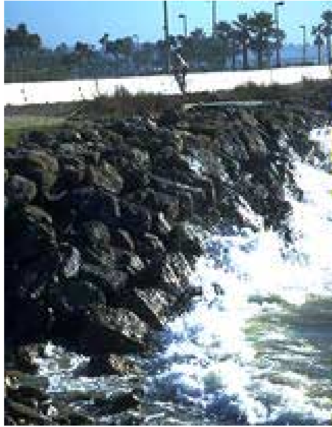
Figure 8. Unpermitted Emergency Revetment at Surfer's Point. [from: http://www.rain.org/~pjenkin/point/point.htm ]
