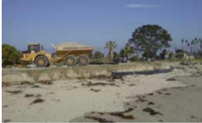
Figure 7. Dredge pipe on beach in front of Goleta Beach County Park. Note large dump truck in the background with sand for the sand berm. [Photo: Shawn Kelly, November 30]
