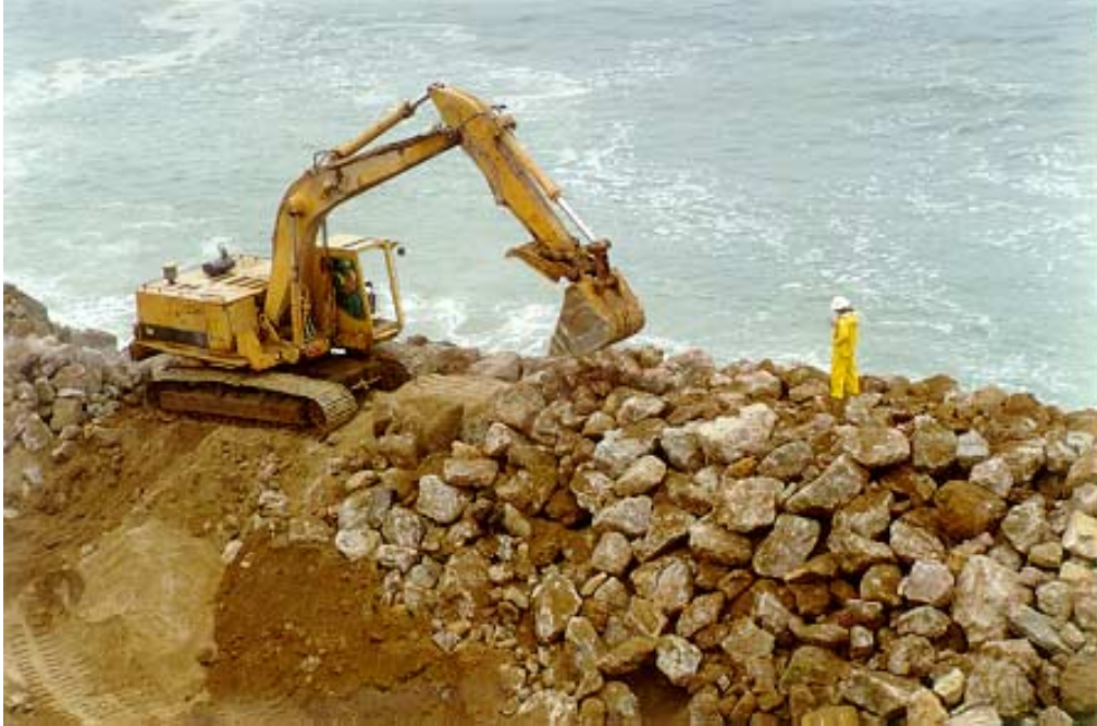
Figure 2. Seawall Repairs, including increasing the seawall height, at Point Mugu, California. Note the complete loss of beach on the seaward side of the seawall. [Photo: Shawn Kelly].
