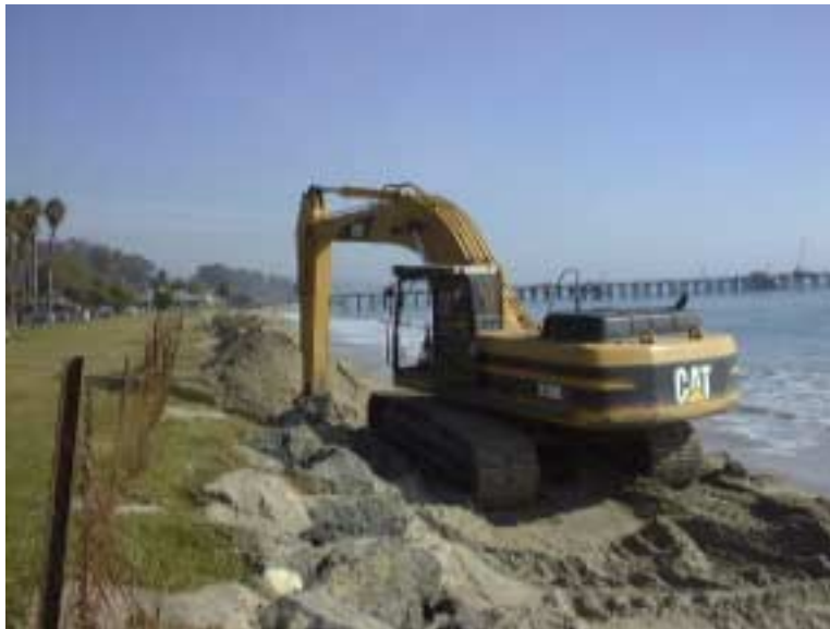
Figure 6. Seawall being removed at in front of Goleta Beach County Park, looking west. [Photo: Shawn Kelly, November 30]
